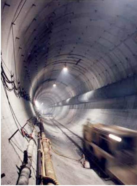
Tunnel Boring technology is more predictable and efficient, and far less disruptive, than the Cut-and-Cover method used for the Central Artery Project.
